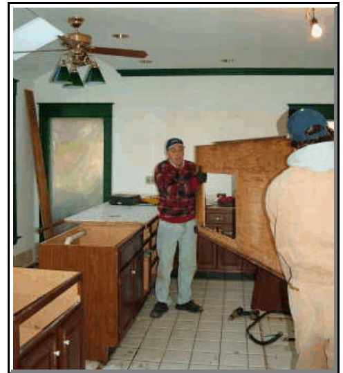
Dennis Eads and Bob Schmidt carry out a worn ceramic tile countertop as my old kitchen is demolished. PHOTO CREDIT: Tim Carter
