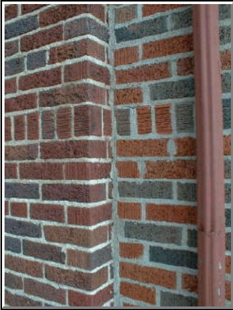
Here is a huge mistake. They matched texture perfectly but the newer brick on the right has too much orange in it.
